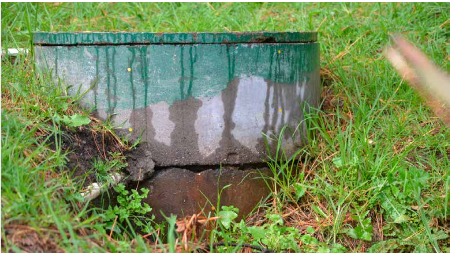
Auckland Council is cracking down on failing septic tank systems.
